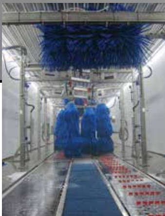
When a car enters the bay, the sensors turn the lights up to full brightness.
